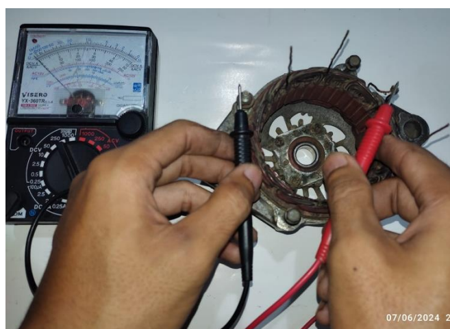
Gambar 14 Pemeriksaan Ground Stator Coil
